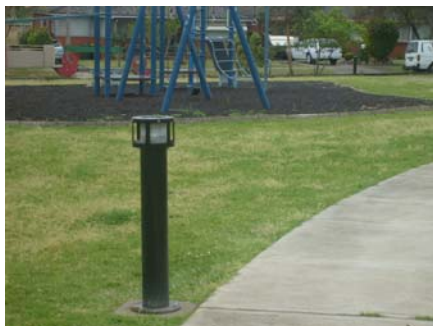
2.29 Lighting near Playground
