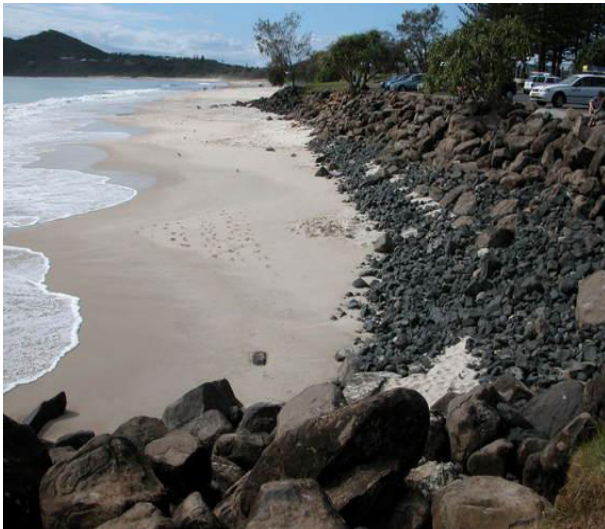
Figure 8: A section of Byron Bay sea wall made of rocks and rubble. (Source: Author 2009).
